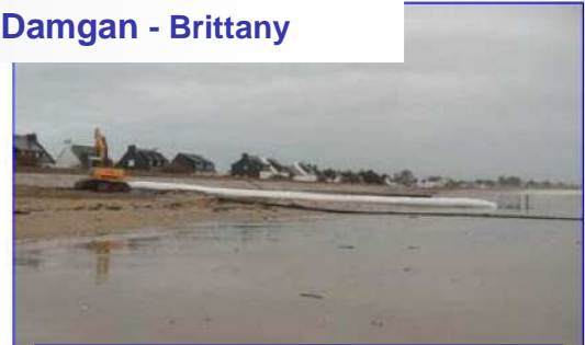
November 2006: End of implementation of two works STABIPLAGE® on the Great Beach of Damgan
