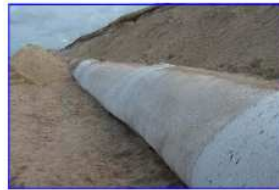
Kerlouan: sight in length of the STABIPLAGE® set up at the bottom of the dune before the phase of reshaping of the front dune.
